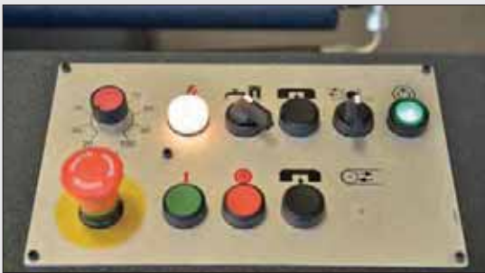
PIC: CONTROL PANEL
