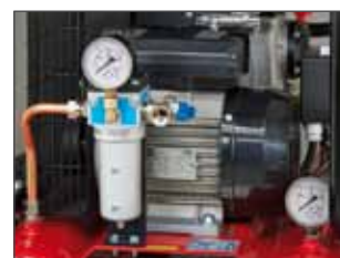
Comandos protegidos contra impactos acidentais. Controls protected against accidental impact.
